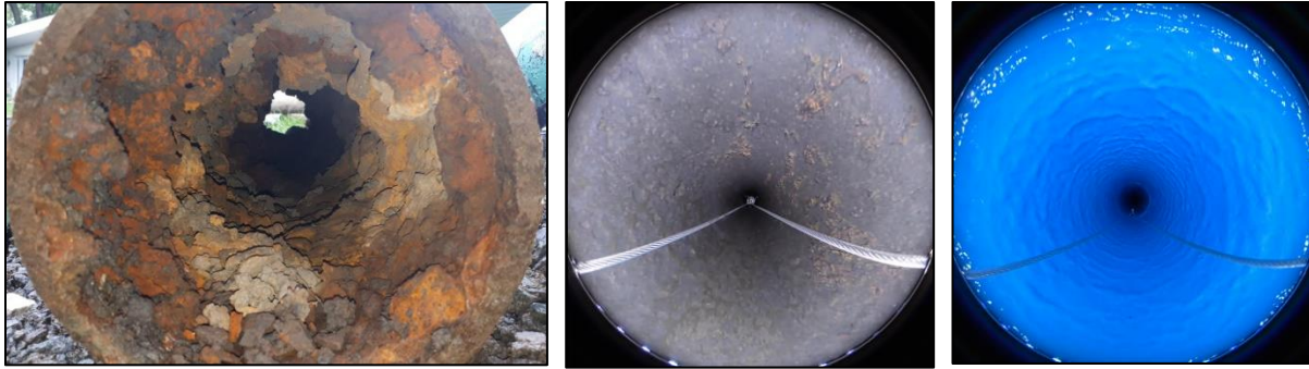
Pictures: Above left, watermain before cleaning, center, after cleaning with Tomahawk, right, after lining with BluKote™.
